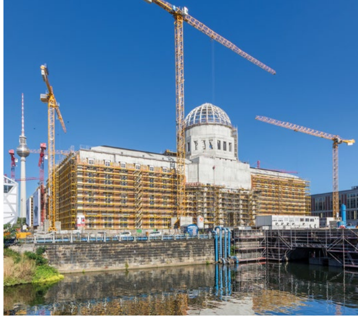
Kieback&Peter are currently equipping the entire Berlin Stadtschloss with building automation systems.
